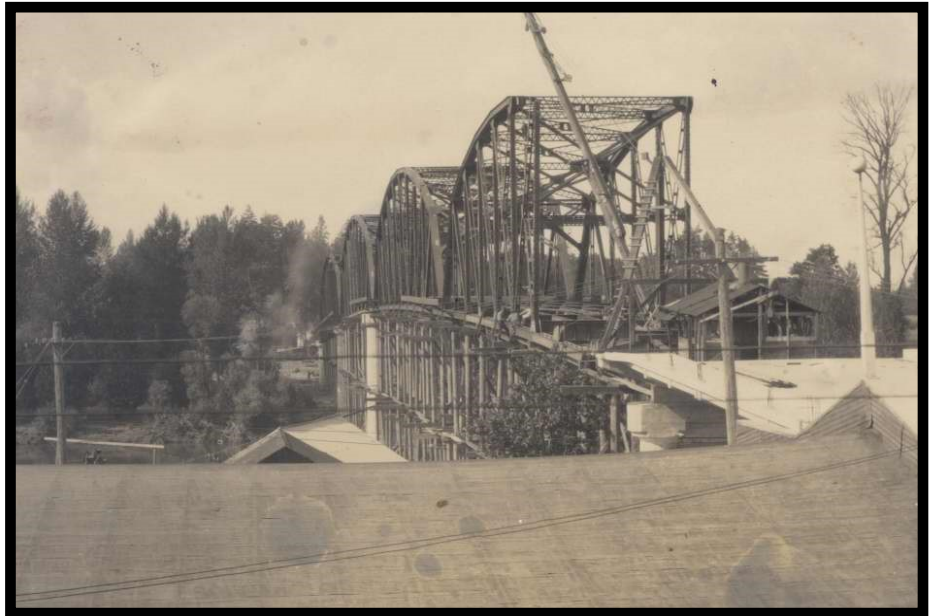
Postcard with photograph on front which shows a view of the Ellsworth Street bridge under construction circa 1925. Museum Collection #1987-012-0001.
